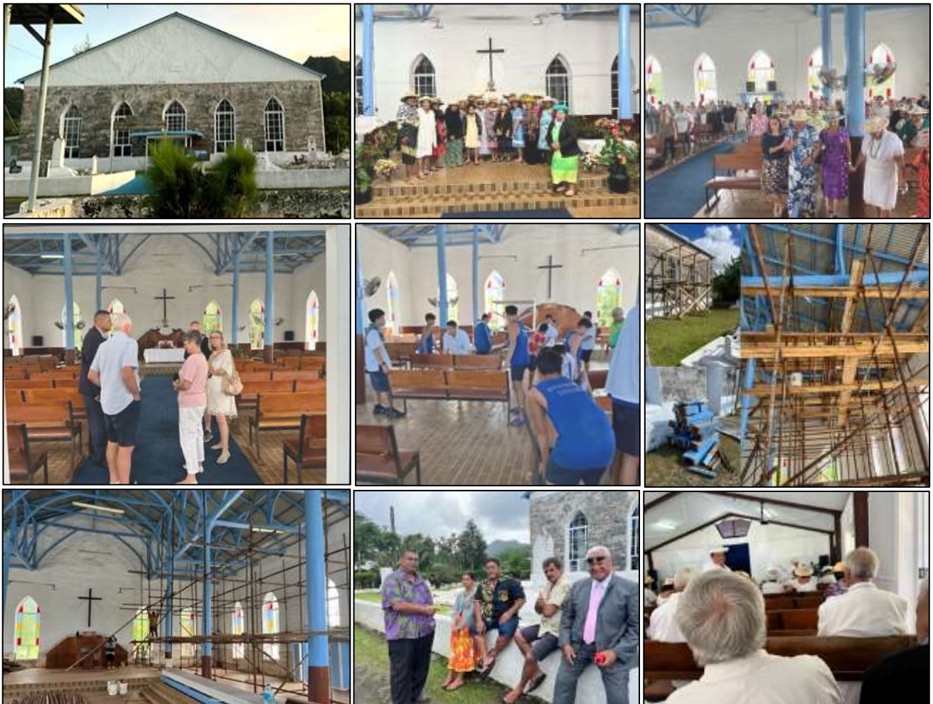
Renovation to BETELA, the Titikaveka branch of the CICC. The Ekalesia is currently holding services in the Sunday School Hall across the main road.
