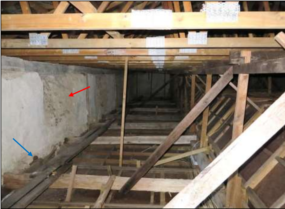
Figure 16: Existing ceiling void. Note the infilled windows from the lowering of the walls c.1944 [red arrow], and redundant wall penetrations for original beams, subsequently removed [blue arrow] (Source: author’s collection, 2014).
