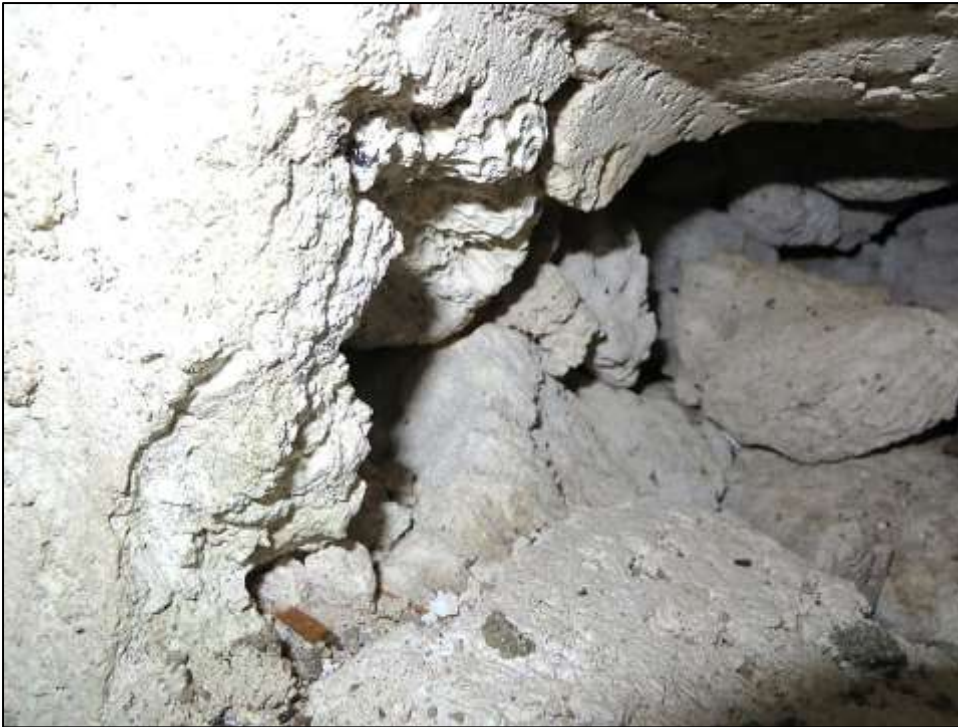
Figure 20: Relatively minimal depth of mortared stonework on the face of rubble (Source: author’s collection, 2014).
