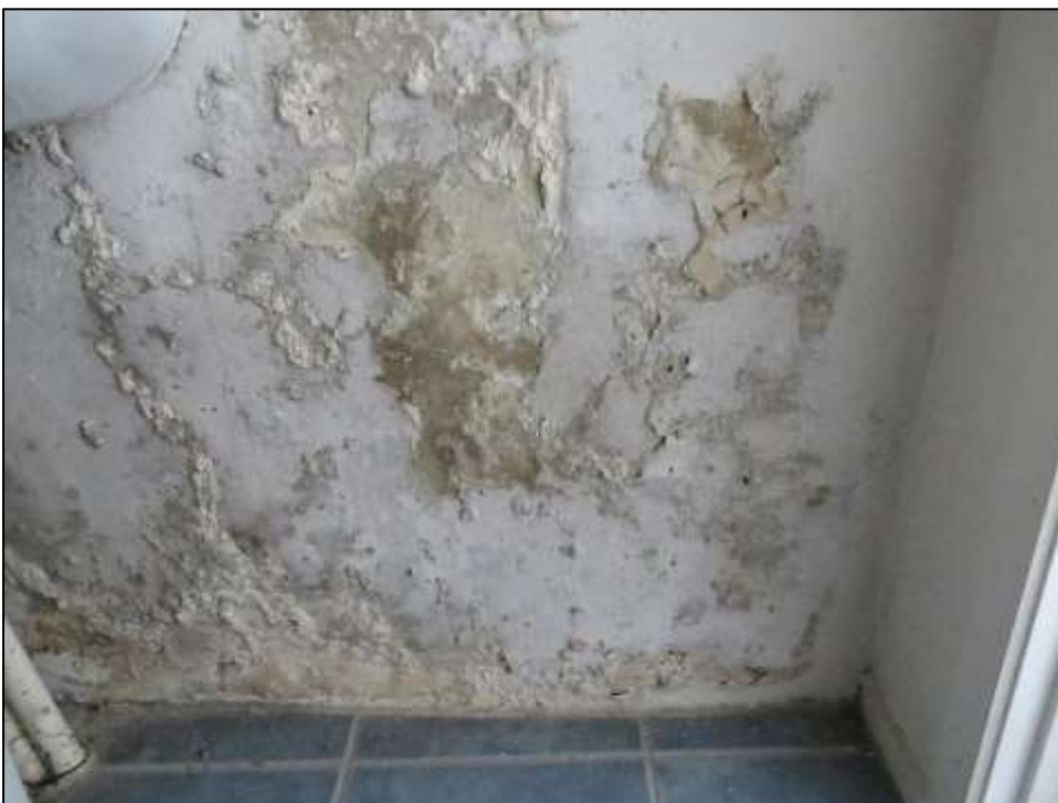
Figure 19: Efflorescence caused by incompatible coatings. This is in the Takamoa Theological College (Source: author’s collection, 2014).
