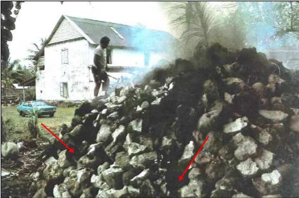
Figure 4: Burning coral to restore the ariki palace in Arorangi. Note the lighting ports [red arrows] which would later act as fire vents. Image © James Siers, photographer (Source: Siers, 1977, p. 95).
