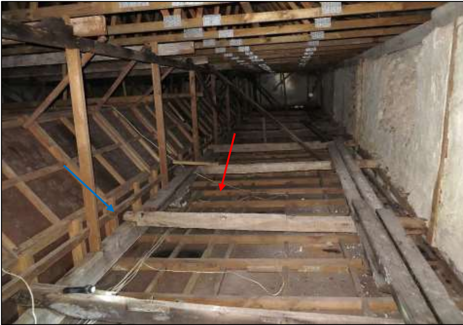
Figure 8: Transverse beams [red arrow] notched onto longitudinal main beam [blue arrow]. Notches are either timber-pegged or mechanically-fixed (Source: author's collection, 2014).
