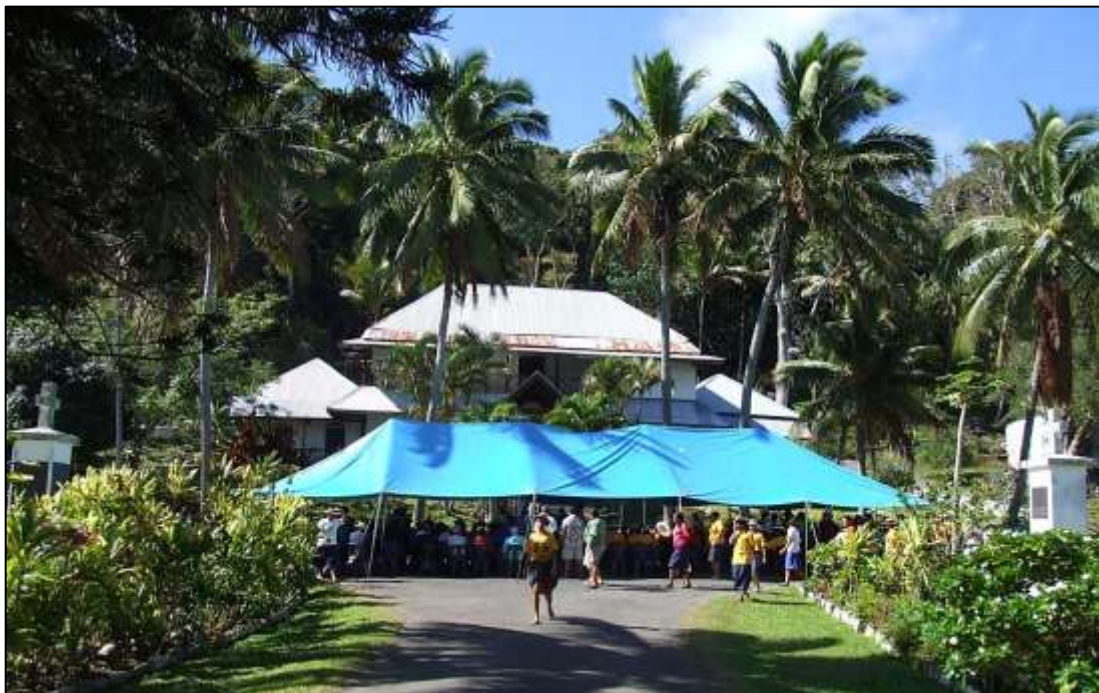
A beautiful day back in September 2008 when a special service was held in front of the old Takamoa Mission House for the commencement of major renovation to the building to become the CICC's new head office. The project was completed and dedicated one year later in October 2009. Photo by the CICCGS.
